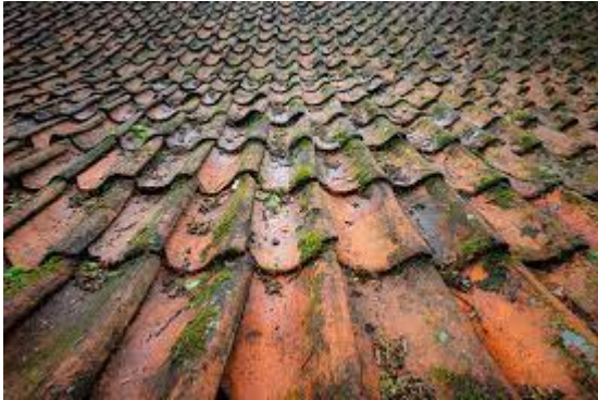
Moss growing on a roof.
